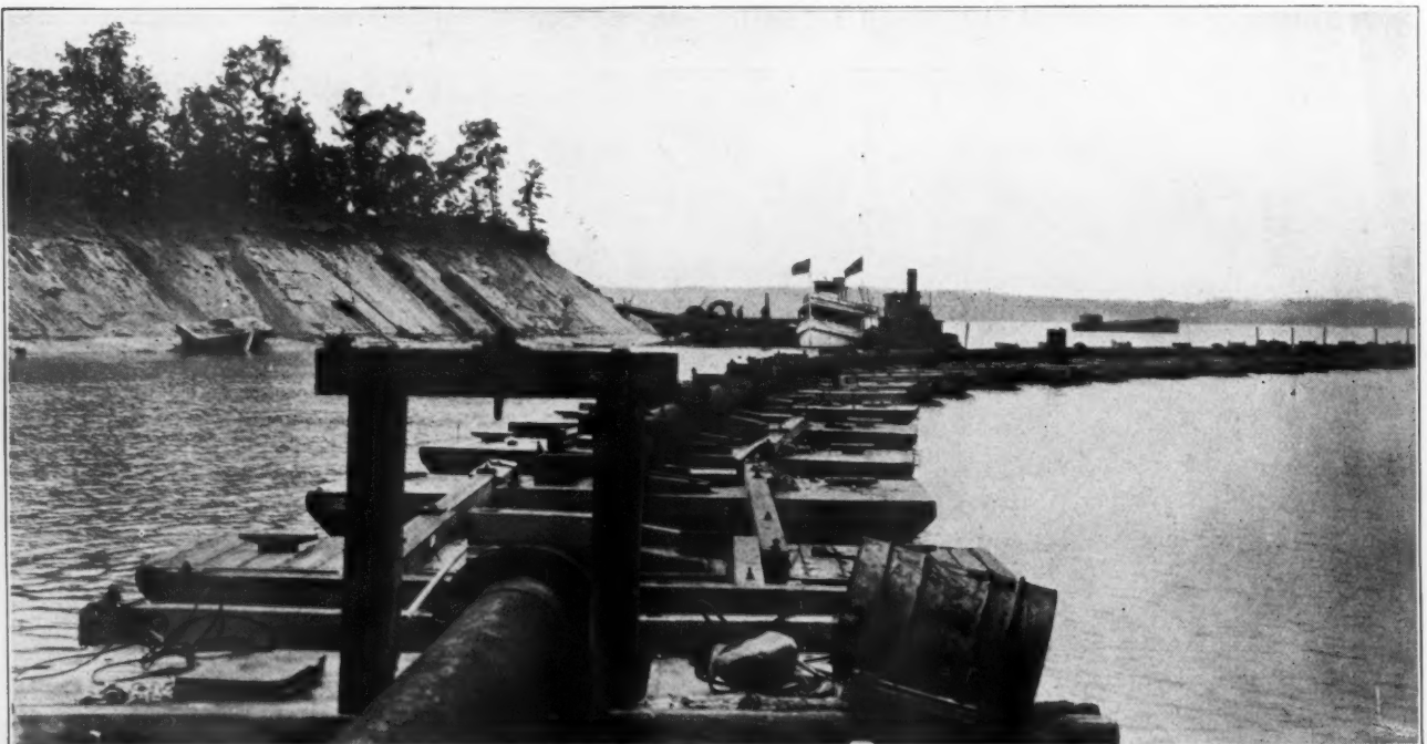
Pipe Line Supported on pontoons
